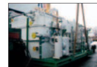
Lubricating oil unit for compressor station with BOLL Duplex filter type BFD-P
