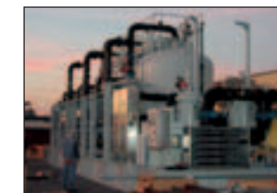
Produced water unit with BOLL automatic filter type 6.18, grade of filtration 50 micron
